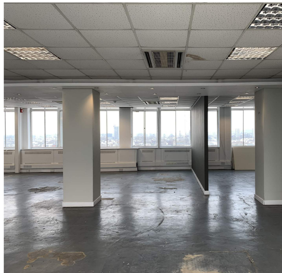
Fig 2.8: Existing view of a typical office floor to Newcombe House after vacant possession
