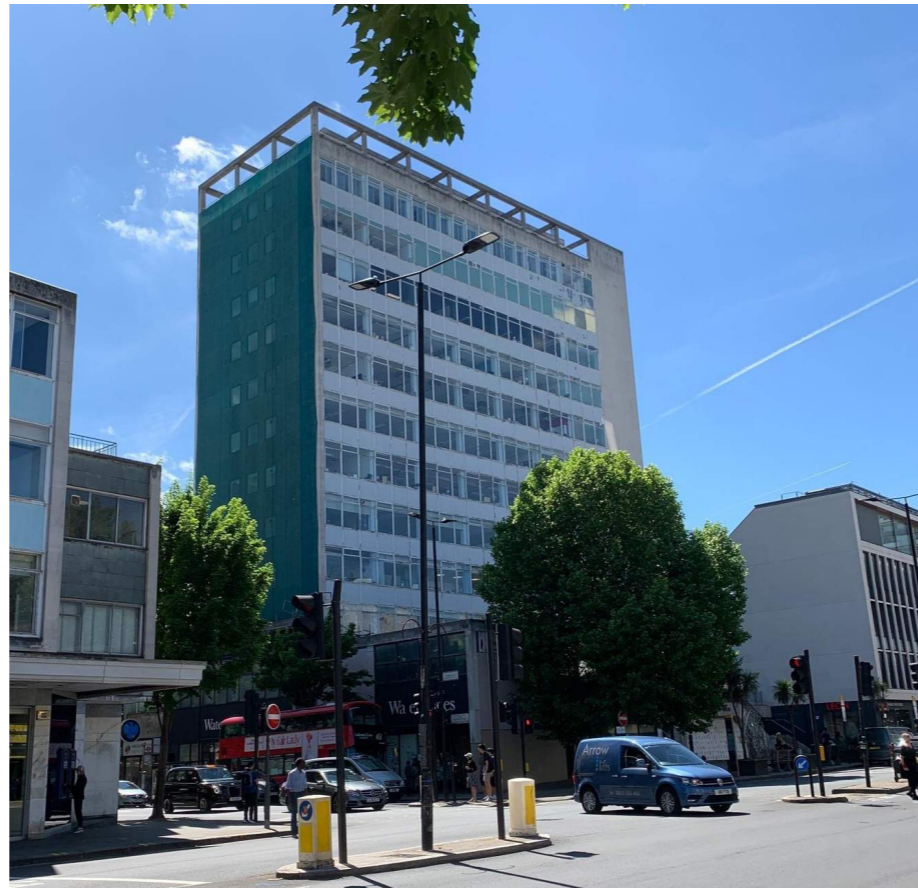
Fig 2.6: View of the protective netting to the east elevation from Notting Hill Gate
