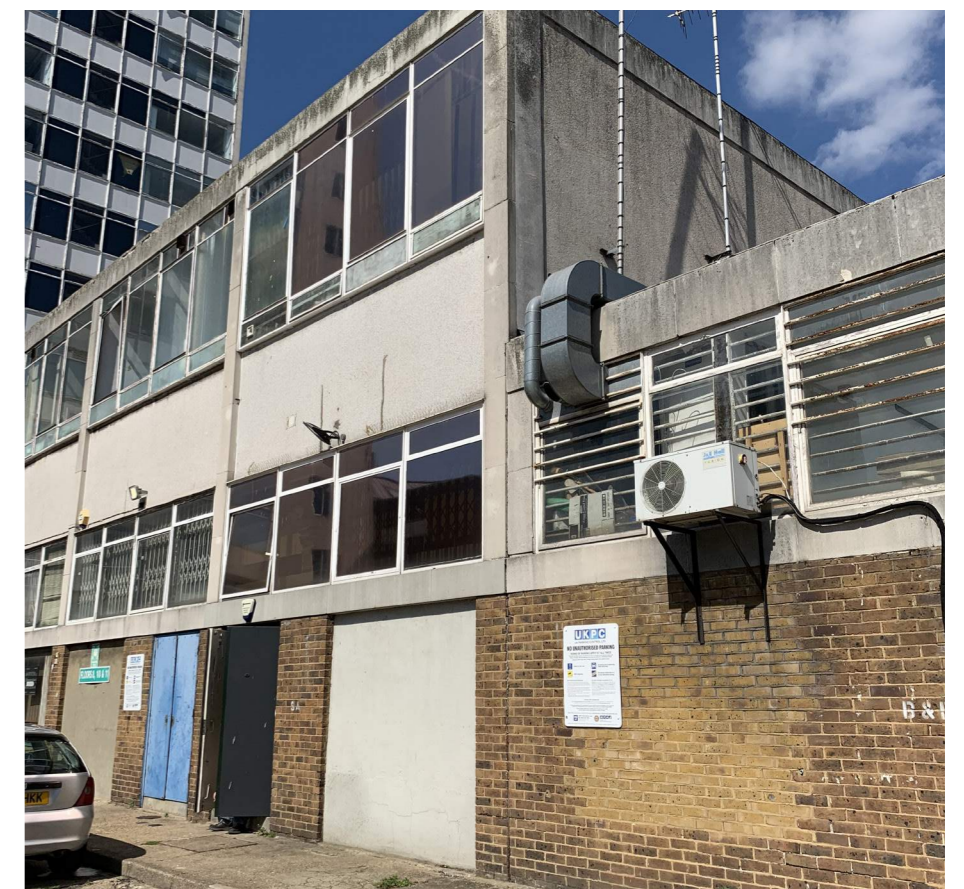
Fig 2.12: Existing view of AC and mechanical plant clutter to rear of retail units
